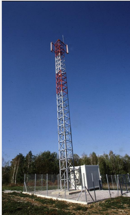
Project: Brdo Radoš Location: Croatia Investor: Ericsson NT d.d.
